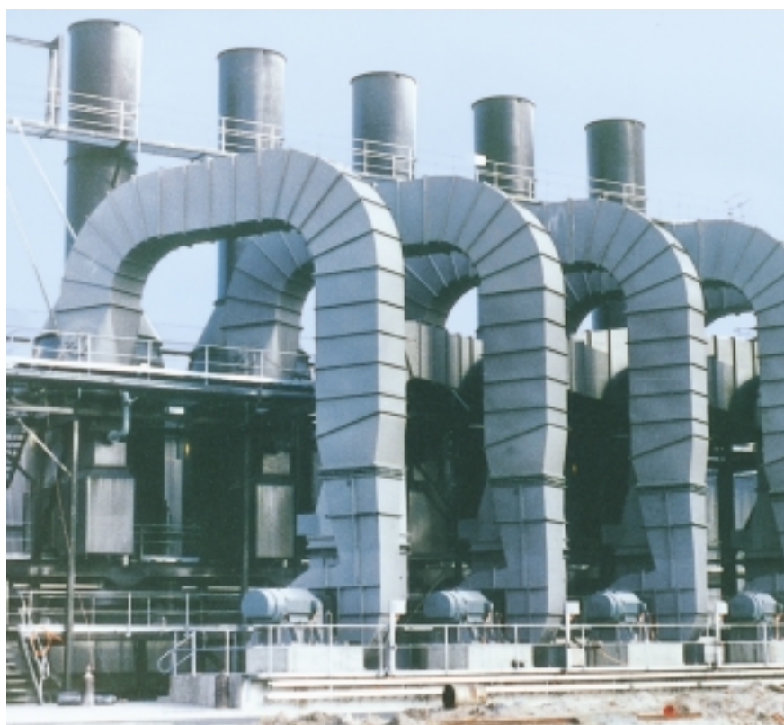
Scrubbers on aluminium pot lines (Australia).
