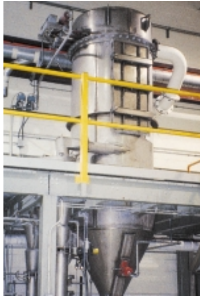
Typical custom built process filter
